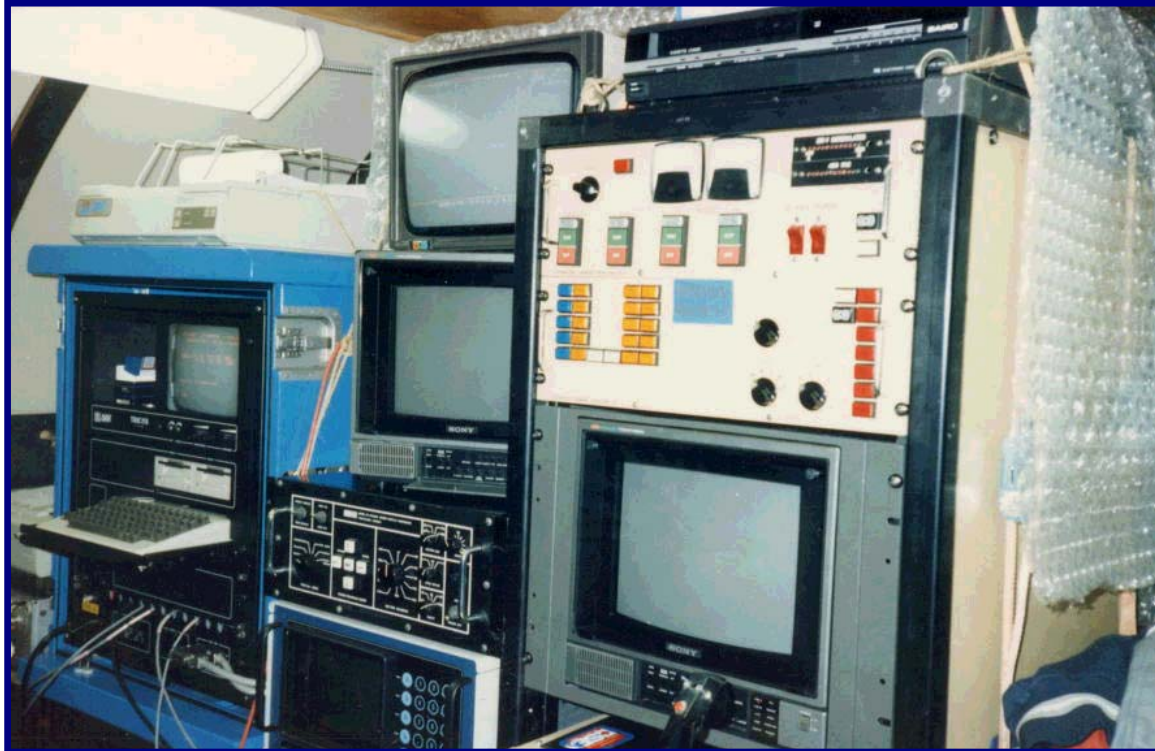
CONSOLE SUITE INSIDE OF SHIPPING CONTAINER
